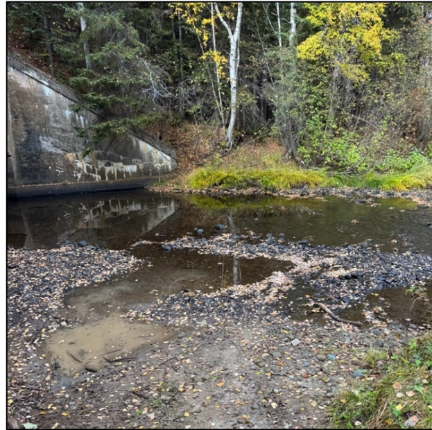
Figure 12 Low water flow and sedimentation occurring at Tabusintac Hill site on Tabusintac River in the fall of 2025
